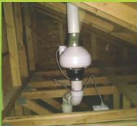
Radon fan installed in an attic.
