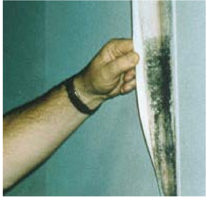
Hidden mold growing behind wallpaper.
