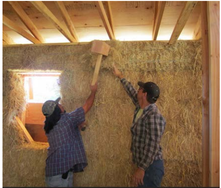
The Pinoleville Pomo Nation built straw bale housing and provided training tribal members and other local tribes' members. Photo: Timonie Hood
