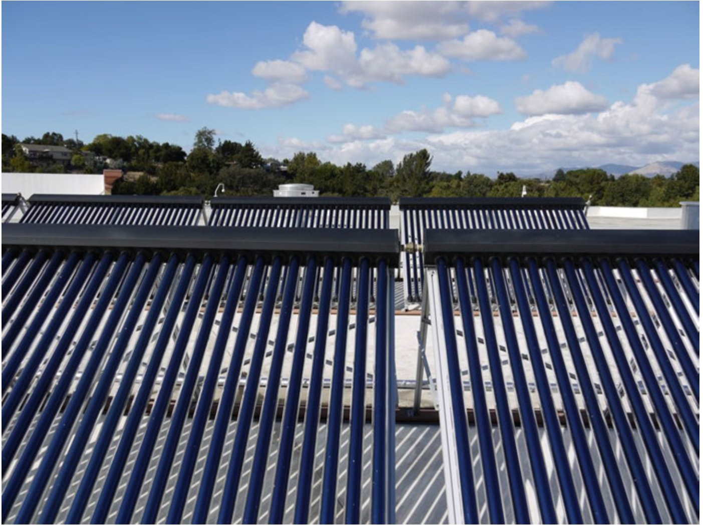
Santa Ynez Band of Chumash Indians in California: Solar thermal system on top of Chumash Casino Resort
